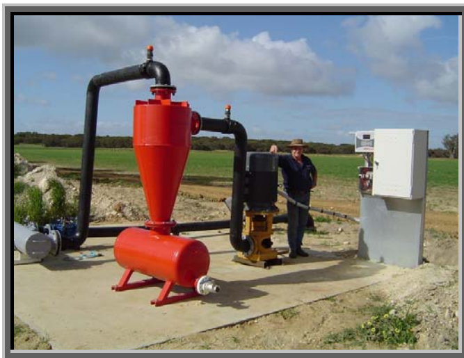
Bore pump and filtering system with computer control panel. Telemetrics back to farm office. (Photo: Mark Stanley)
