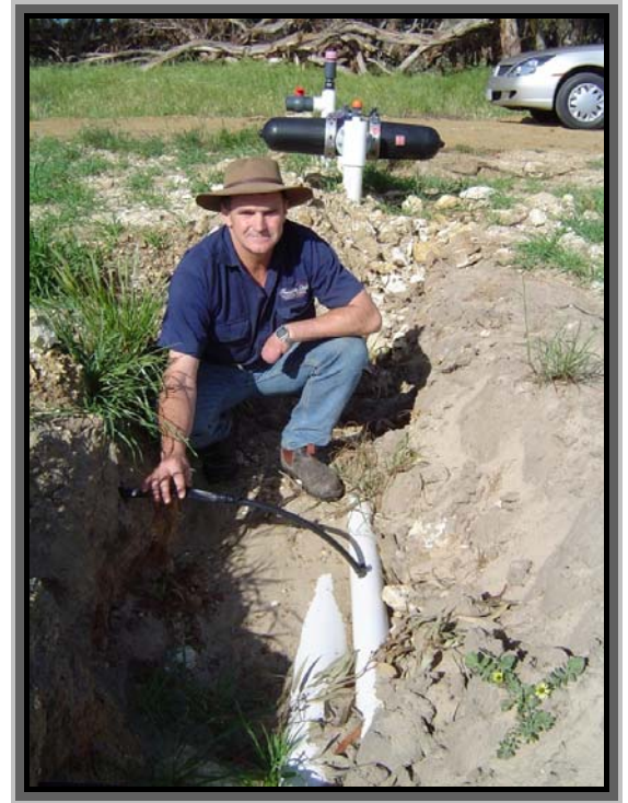
Brendon Smart with sub-surface drip line..(Photo: Mark Stanley)
