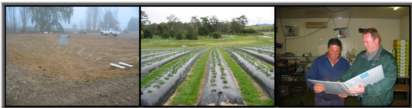
Construction of a sediment trap which will reduce strawberry property nutrient run off, and provide nutrient recycling options for future strawberry crops
